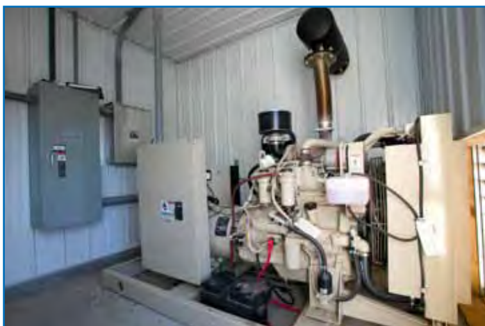
Figure 100: Example of a back-up generator.
