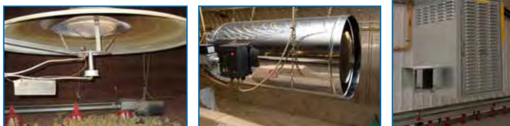
Figure 101: Examples of different house heating systems (from left to right, canopy brooder, whole-house heating, and space heater).
