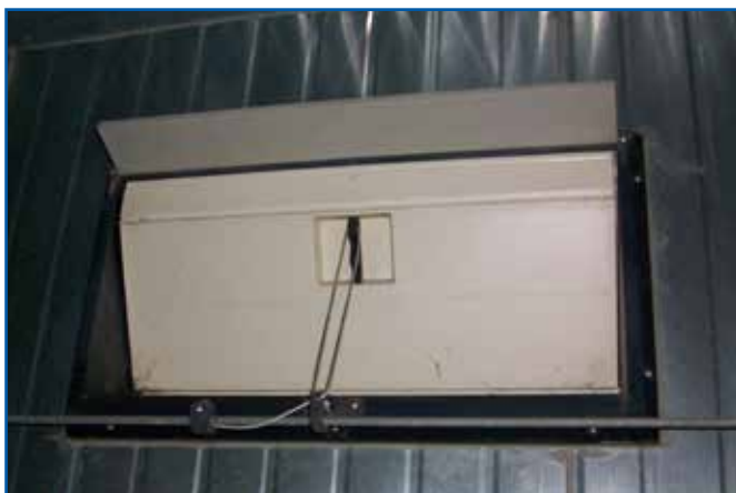
Figure 6.9: Example of a good-quality air inlet.
