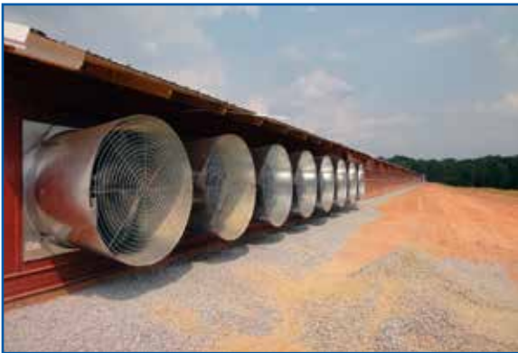
Figure 6.13: Example of a typical tunnel ventilated house.
