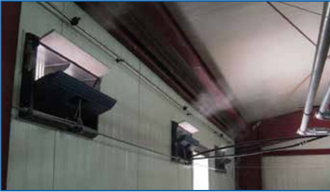
Figure 6.21: Example fogging system for a cross-ventilated house.
