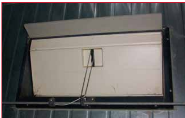
Figure 6.9: Example of a good-quality air inlet.
