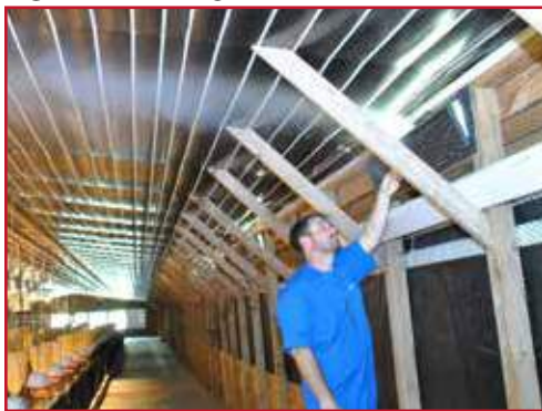
Figure 6.7: Using a smoke test to determine if airflow and operating pressure are correct.
