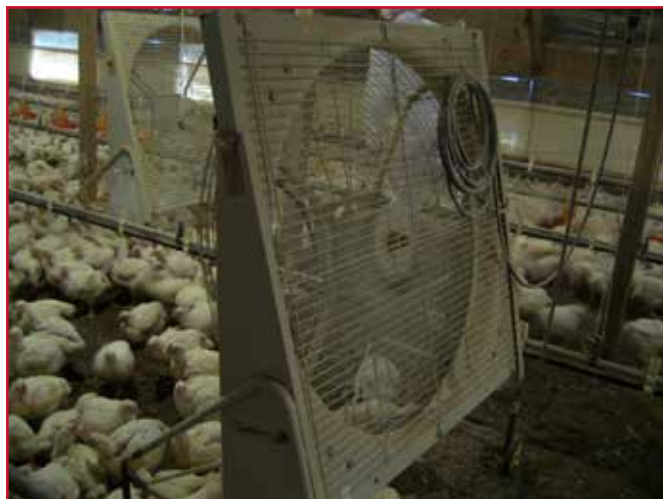
Figure 6.2: Circulation fans in a naturally ventilated house.
